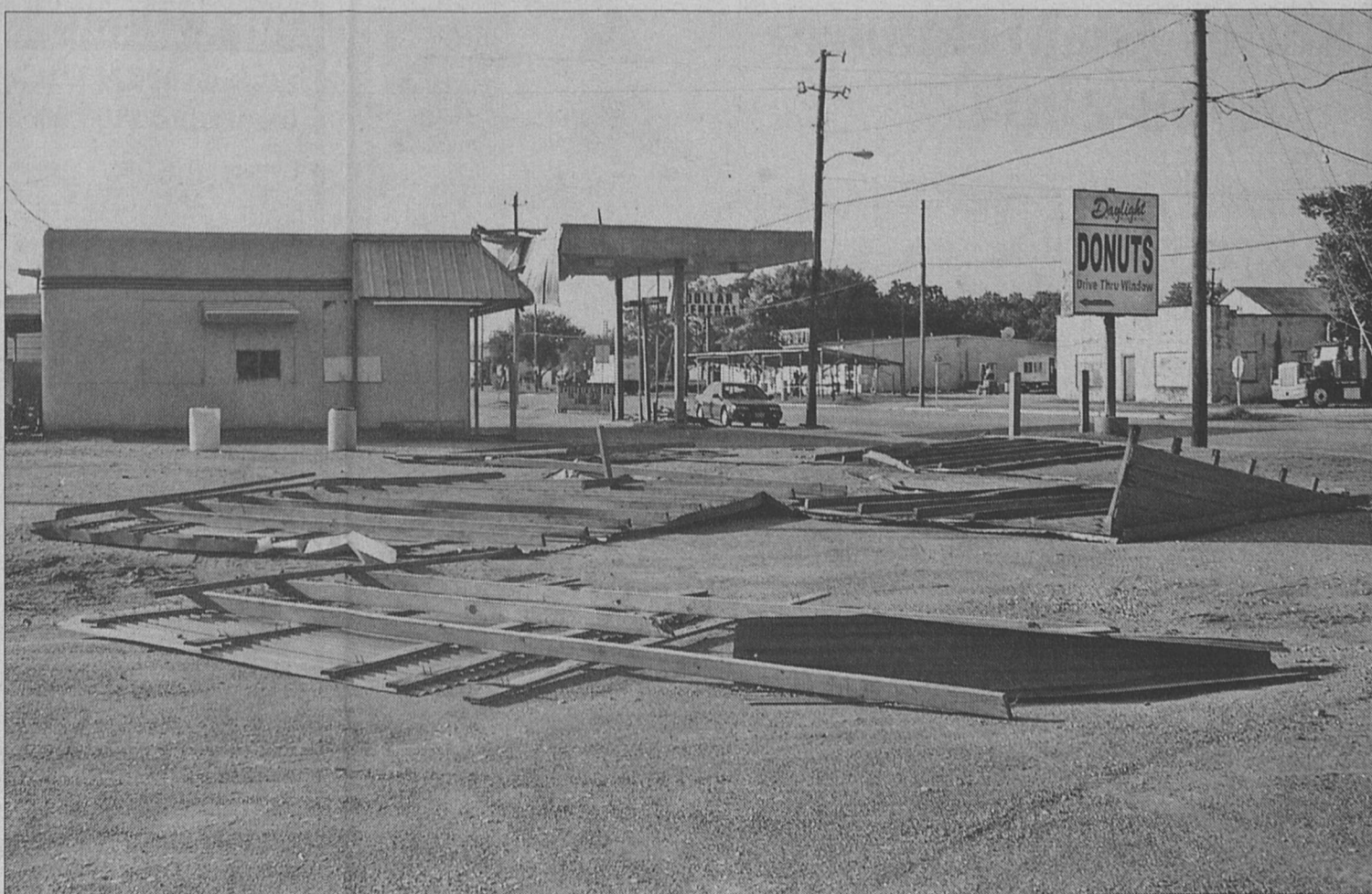
On Sunday, August 3, a wind gust blew a good portion of roofing material off the top of the Daylight Donut Shop here in town. There were some reports of a small twister or tornado-like wind from witnesses nearby.
