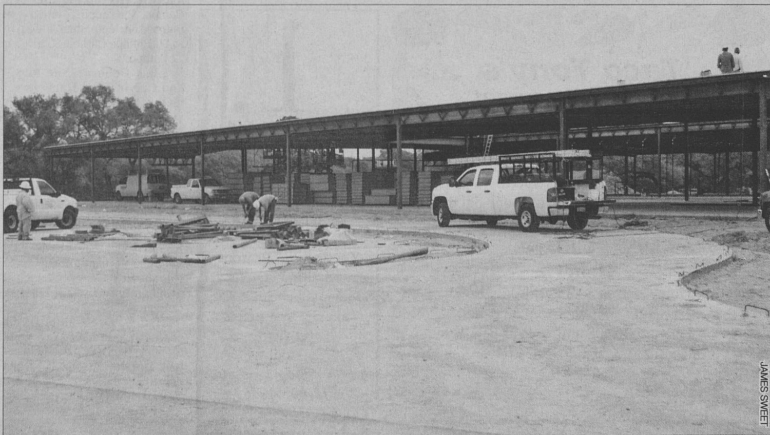
Work continues on the new Junior High Facility in Altair. Crews also started on the ground work for the gym facility recently.
